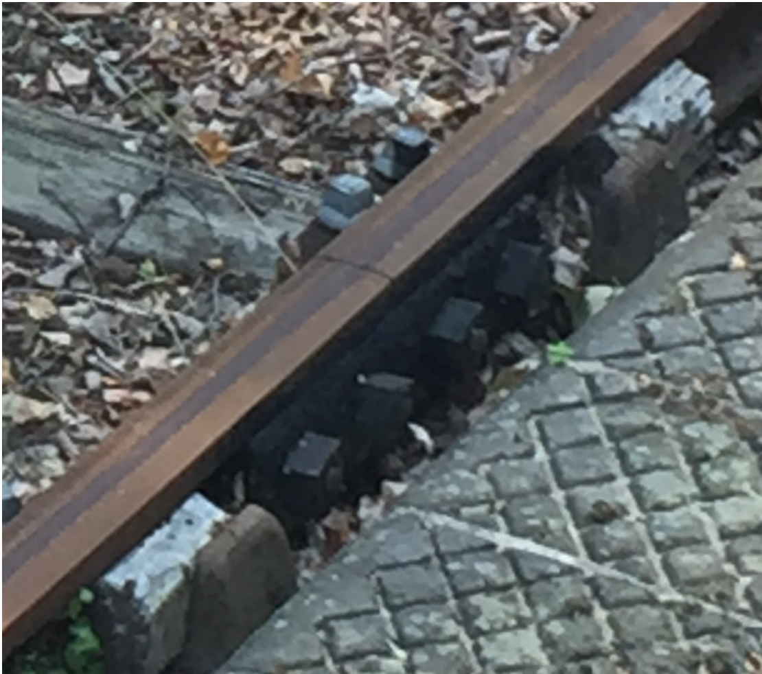
Figure 7 Rail joint near 3 Westward Ho in ambient temperature of 29°C
